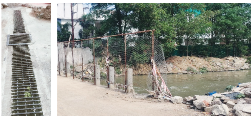
Figure 20. Existing Drainage Network Situation (a) Perforated Design for Drain Covers (b) C&D Waste Affecting Nallah
